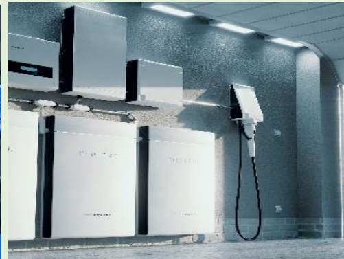
3. EV Charging Station
